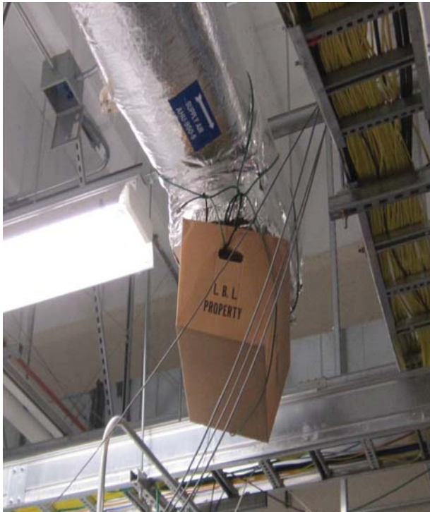
Figure 55 Box being used to avert downward air currents.
