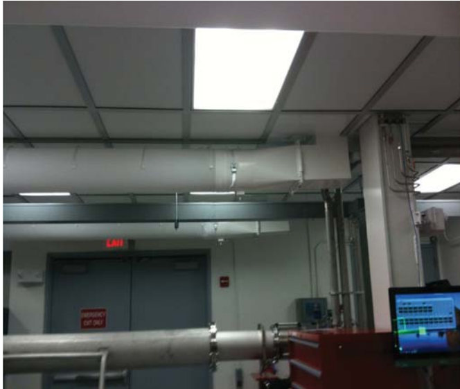
Figure 56 Example of an "Air Sock" ventilation approach.
