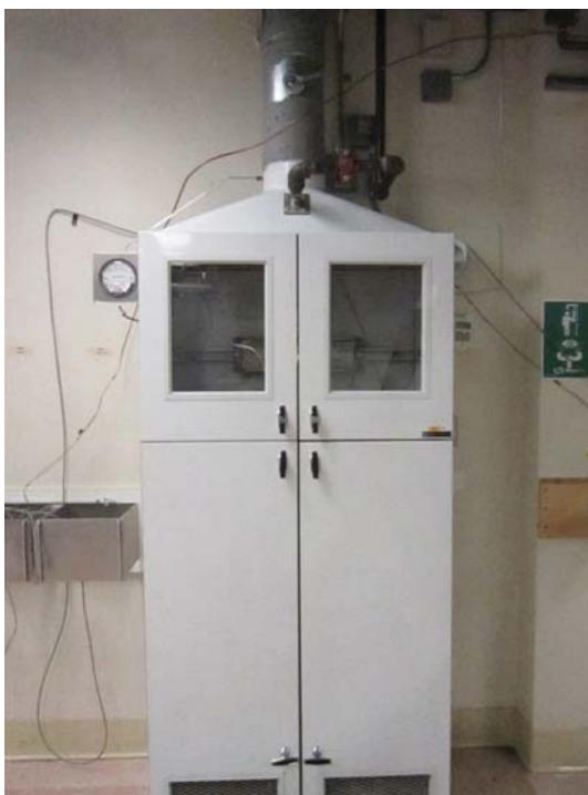
Figure 57 Excimer gas cabinet.
