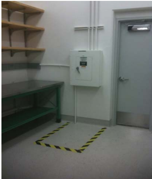
Figure 59 Clear space around electrical panel marked off and clear.
