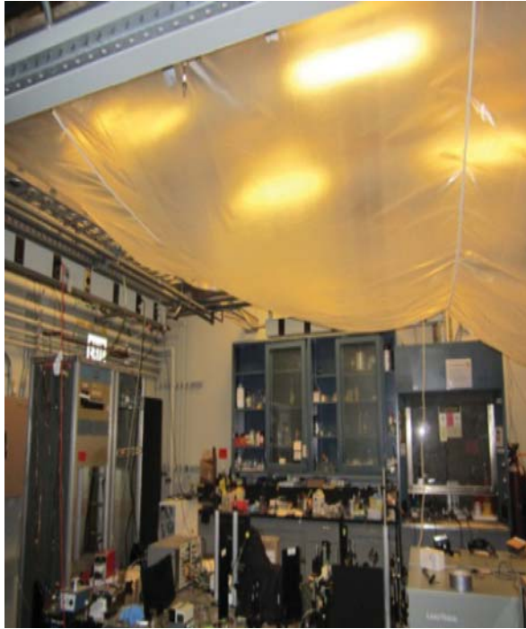
Figure 54 Plastic hanging from ceiling to trap particulates from air handling system.
